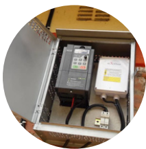
FCH installed solar lighting in 6 houses plus the Administration office, leaving only 2 houses left to be installed.
